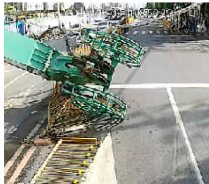
塔吊倒地离公交车车头仅两三米
